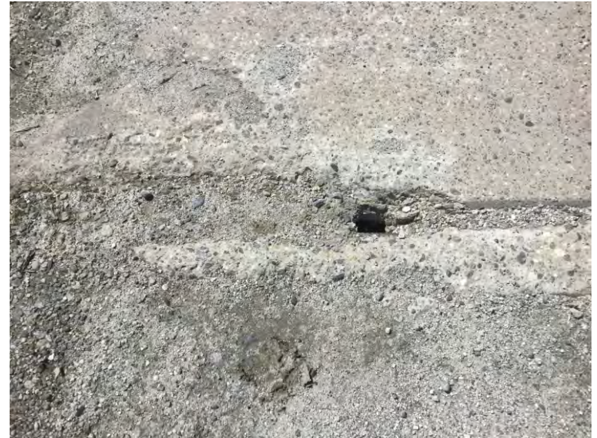
Damage noted to top of right ballast wall
