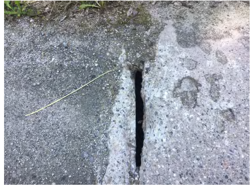
Damage noted to left ballast wall and panel 1
